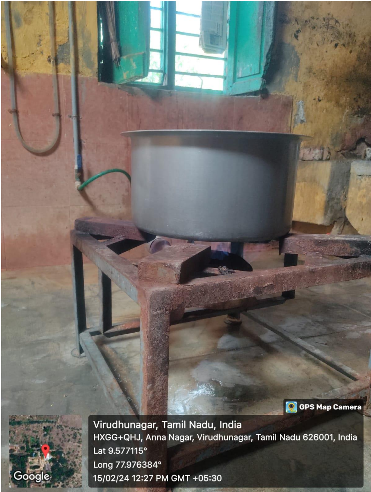
Bio Gas Stove At Boys Hostel Mess Kitchen
